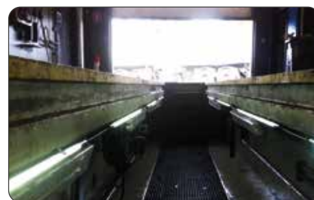
Example of LINE LIGHT solution mounted in a truck mechanic's pit
